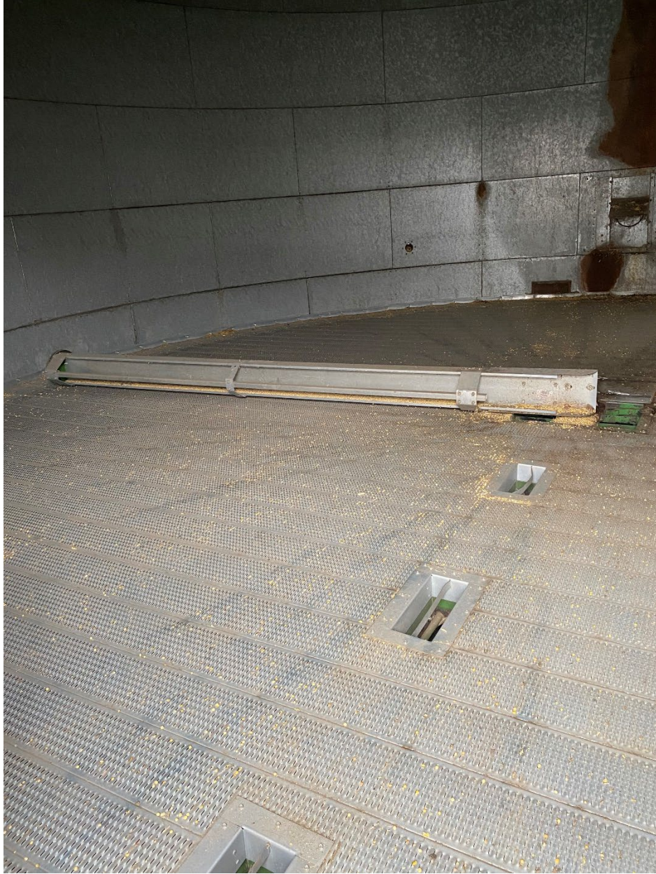
Floor and power sweep inside the 25 foot bin
