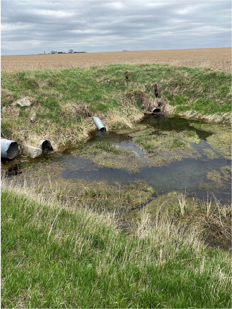
Parcel 1 Tile outlets at the south end (beginning point) of the drainage ditch
