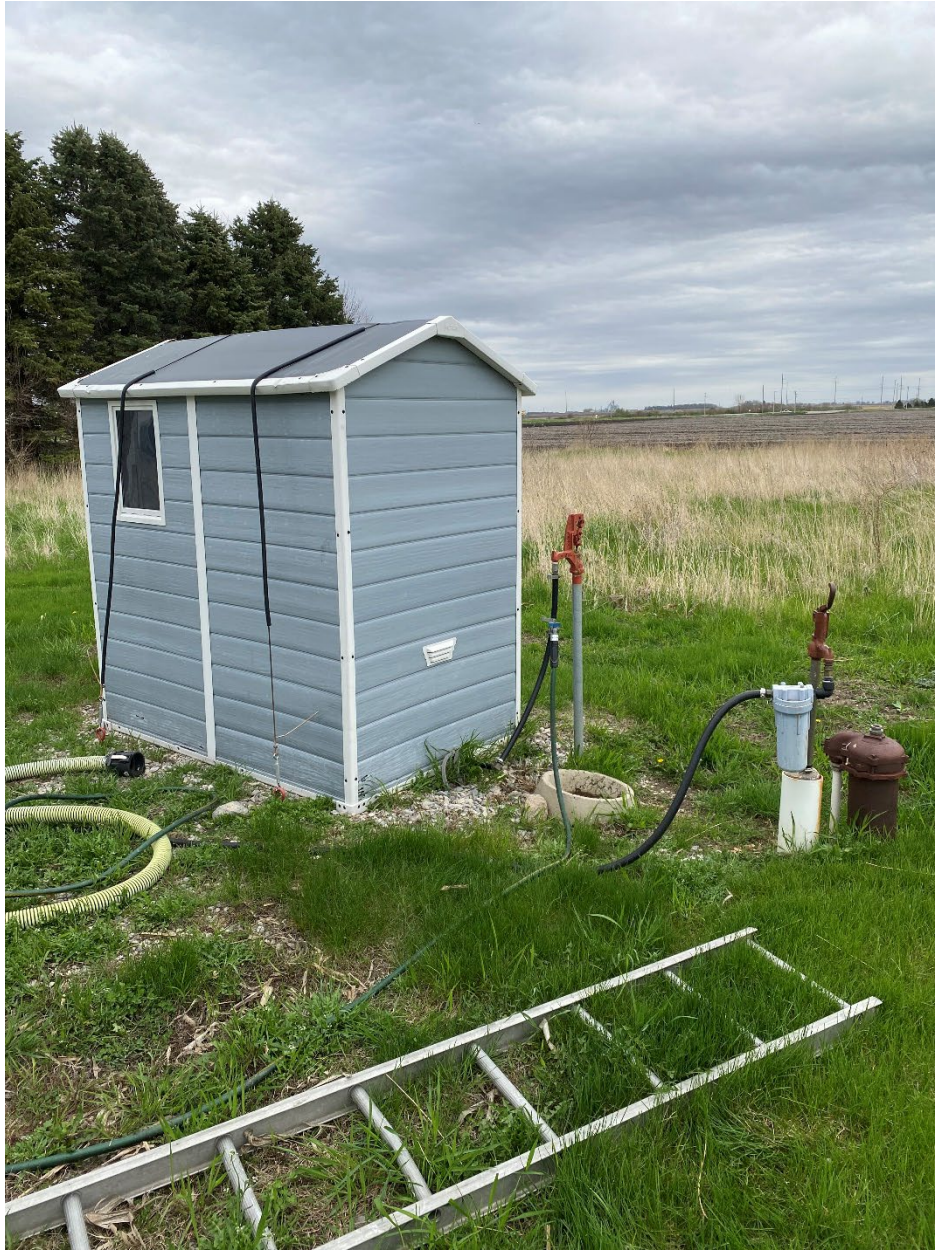
Well and water hydrant. Pressure tank inside shed.
